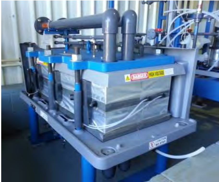
Electrolytic Cell Module
