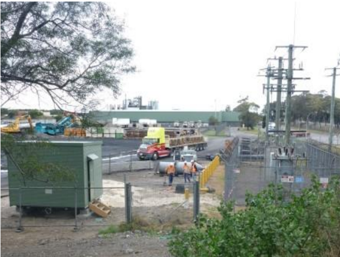
The 33 kVA switchyard and the high voltage switch room. The NIRP is connected to the switch room via a 350m underground cable.
