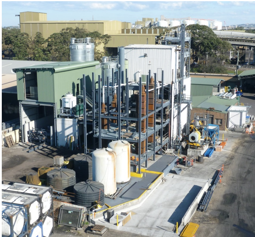
A view of the NIRP from the north. The banded SPL delivery/HCl acid load out area is in the middle foreground, and commissioning of the mill scale preparation area on the western wall of the Plant has commenced.
