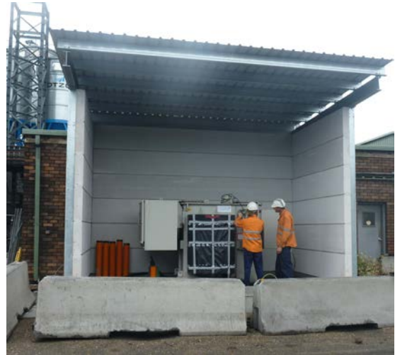
The installation of the 2,000A, 33 kVA transformer and bundled housing is complete.
