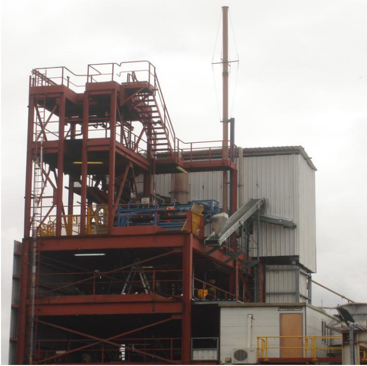
View of Process Tower showing installation of the Vacuum Belt Filter, Ilmenite Conveyors, and Exhaust Scrubbers and Stacks
