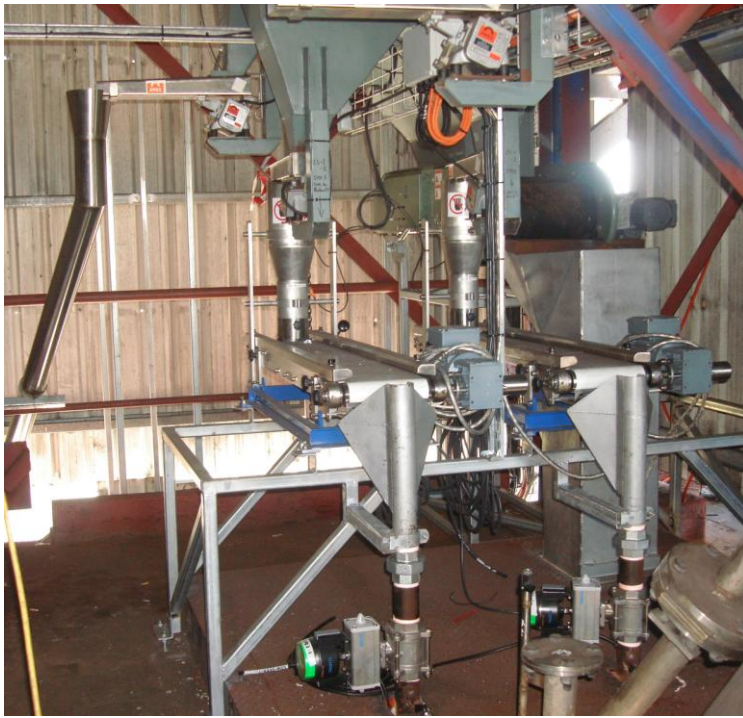
Installed Coal Weigh-Feeders and Roasted Ilmenite feed chute to the Rare Earth Magnetic Separator
