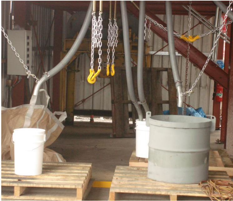
Rare Earth Drum Magnet discharge system. Roasted Ilmenite Product and Non-Mag reject fractions will fill bulker bags on separate weigh scales.
