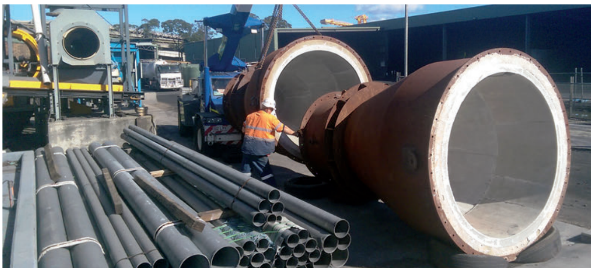
Delivering two fluid bed roaster bodies to be used for gasification in the NZIRP
